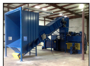
'Walking Floor' Truck Unloading and Baling System
