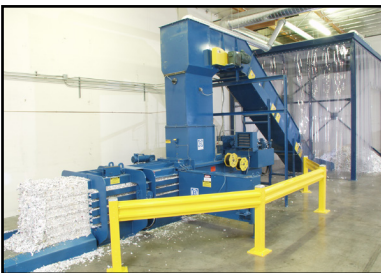
The Original AES Truck Unloading and Baling System
